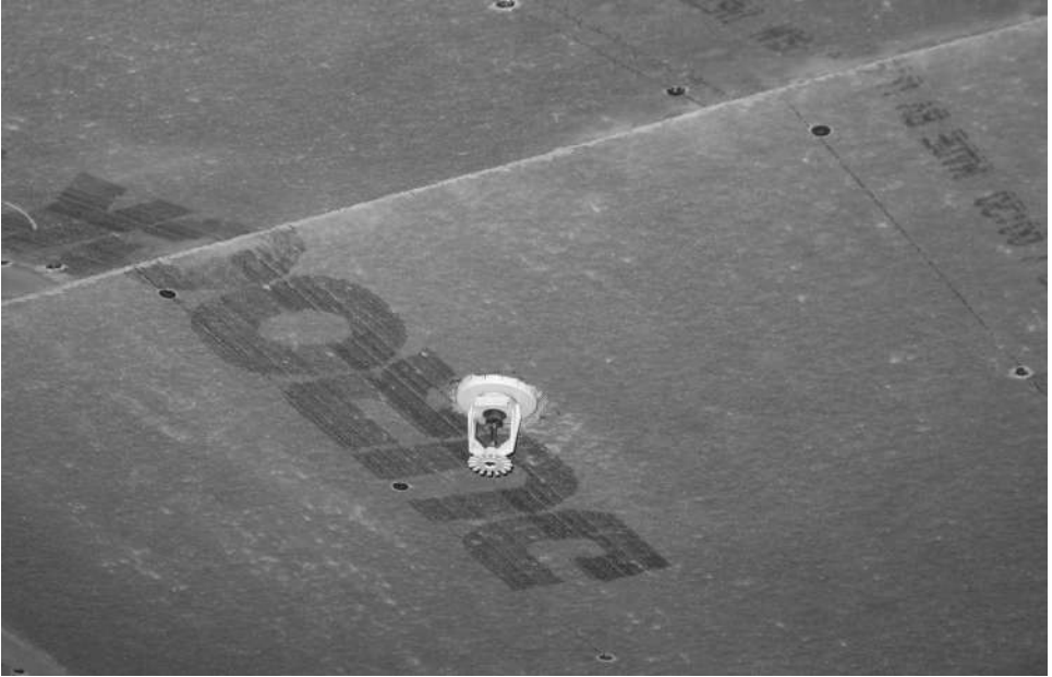
Ceiling (with fire sprinkler head) showing Tile Council of North America (TCNA) recommended pitch of 2" per foot (50mm per 300mm).
