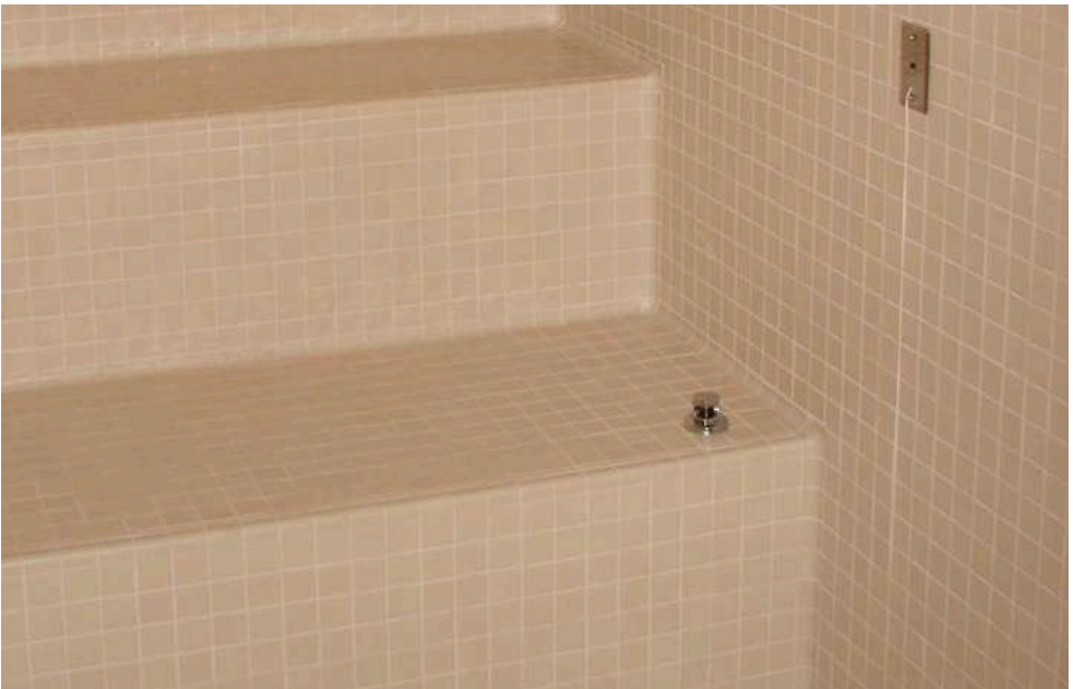
Same view of finished installation after grouting with SPECTRALOCK® PRO Premium Grout and LATASIL™.
