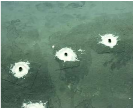
Figure 6.3.5 — Epoxy waterproofing membrane is applied at the pipe penetrations over the cured liquid applied waterproofing membrane to ensure a complete seal at the penetrations.
