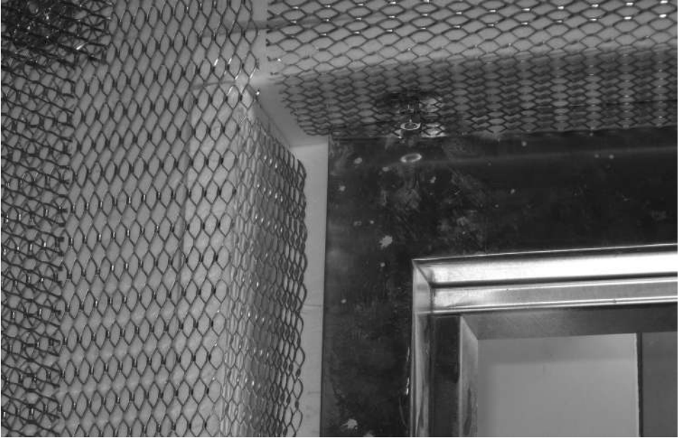
Installation of 3.2# expandable diamond metal lath to stainless steel door frame and flashing.
