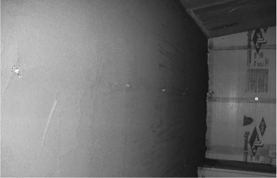
A finished scratch coat wall that is now ready for the float coat.
