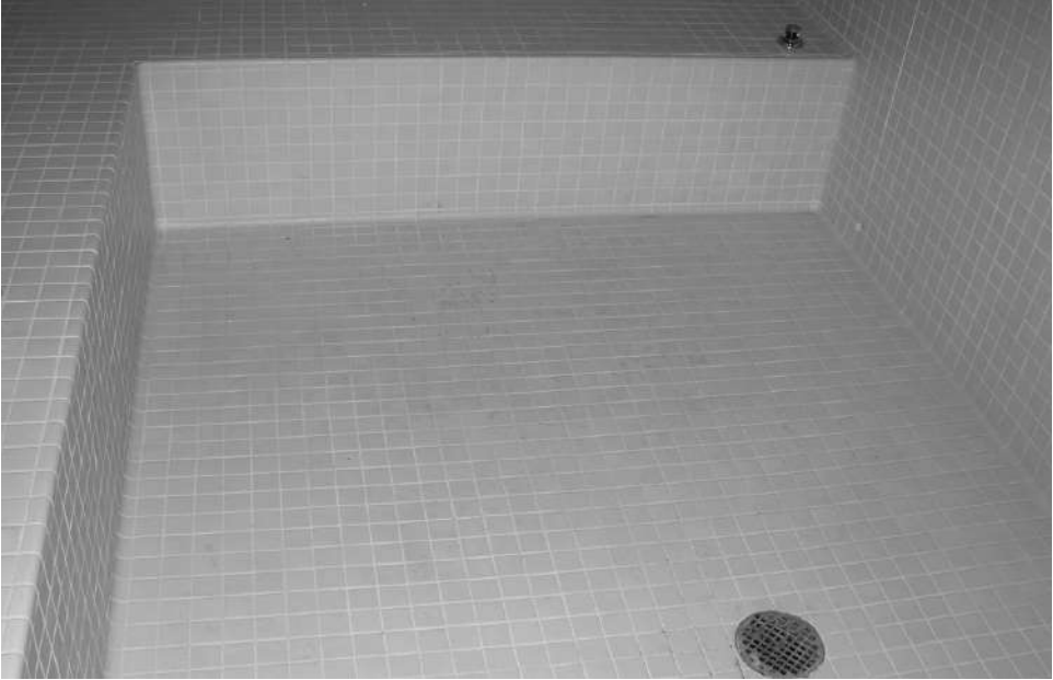
Finished floor installation of tile. Floor and seats are sloped \frac{1}{4} " per foot (6mm per 300mm) to the drain.
