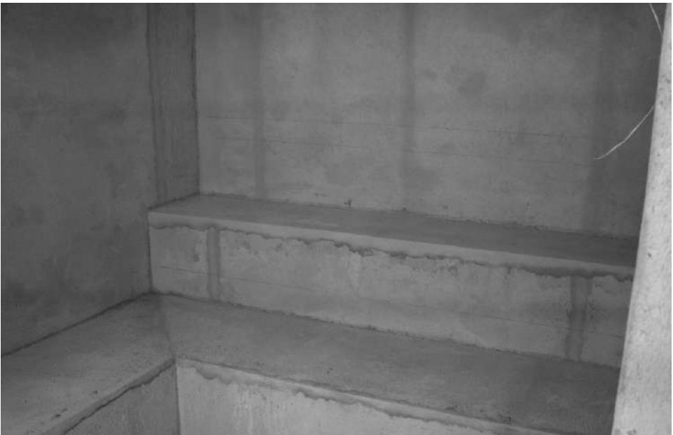
The steam room seats after the installation of the 3701 Fortified Mortar Bed.
