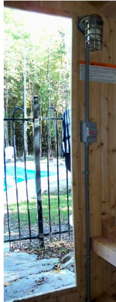
Conduit run inside sauna (Note: customer's own light in picture)
